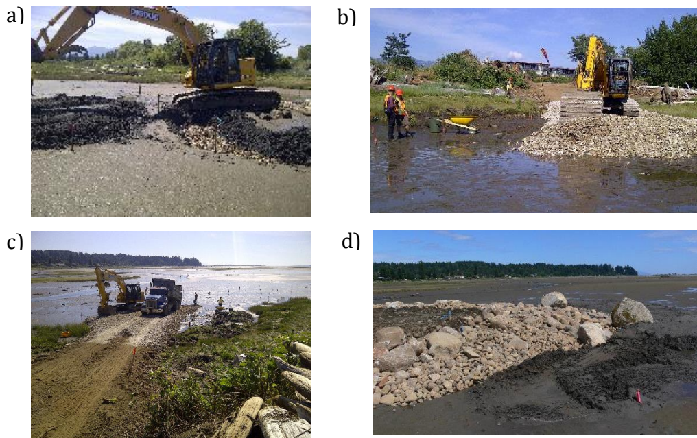
Figure 50. Construction of saltmarsh islands. a) Fill was added to allow movement of heavy equipment onto the mudflat; b) larger rock was incorporated at the front edge of each island; c) construction of the second island; d) detail of the front toe of the second island.
